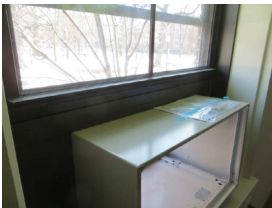
Through-wall AC units in a panel fixed within the window. View from interior.
