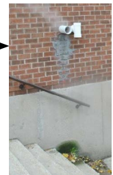
This boiler vent deposits condensate on the wall of the buildings and on the stairs leading to a shared laundry facility.
