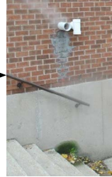
This boiler vent deposits condensate on the wall of the buildings and on the stairs leading to a shared laundry facility.
