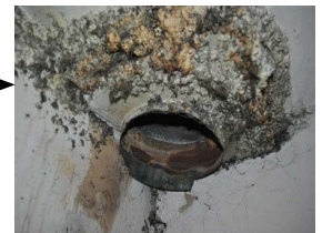
This abandoned exhaust vent provides a direct air leakage path to the exterior. It requires patching.
